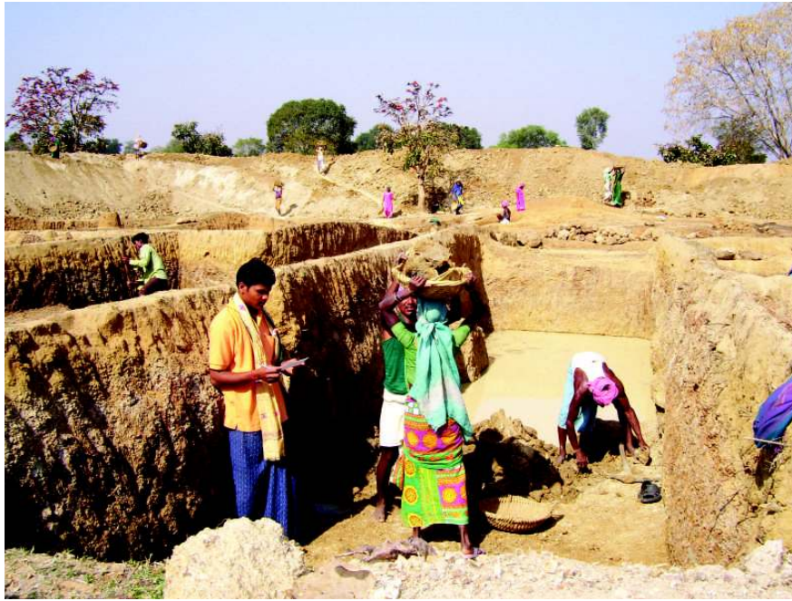
A water harvesting structure (WHS) planned by Jan Mukti Anushthan under construction in Balipadar village of Bankel GP
