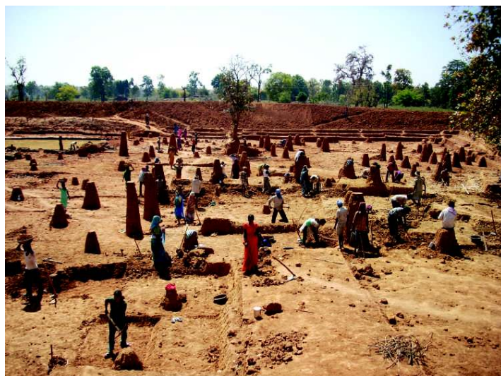
Work on an earthen dam designed with support from Gram Sudhar Samiti in progress in Sidhi
