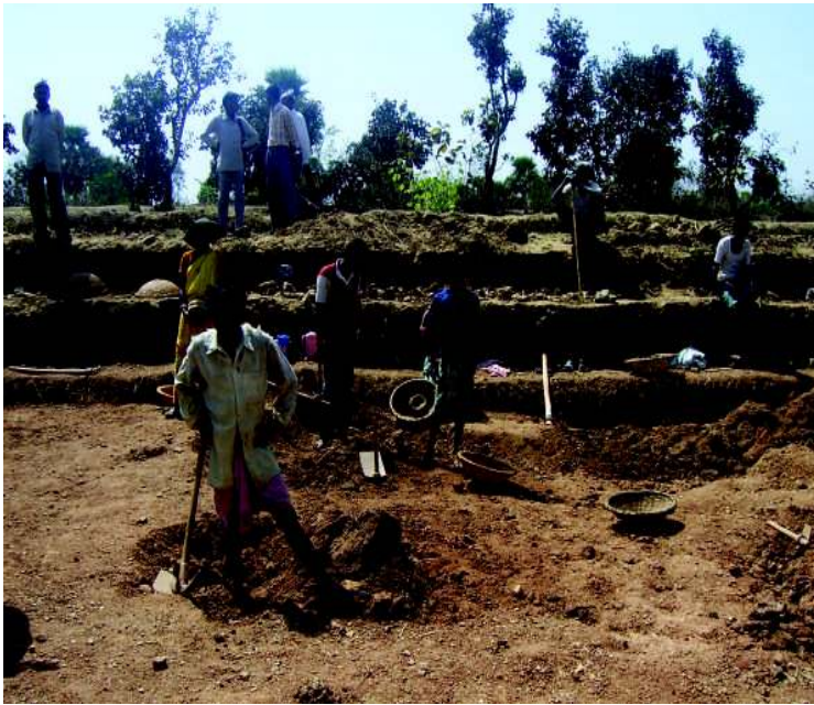
A Hupa under construction. Typically, the 5% model is undertaken by farmers with fields in the mid-level slopes. The farm pond is locally referred to as a Hupa as the depth of a Hupa is 10 feet. After protective irrigation also farmers get enough water in those Hapa to irrigate their second crop
